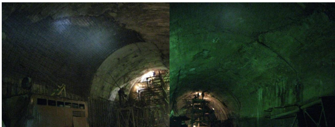
Figure 4-6 : DT2 tunnel, on the left collapsed area downstream of the gate section; on the right cracks on the crown in the stretch between the gates chamber and collapsed area
