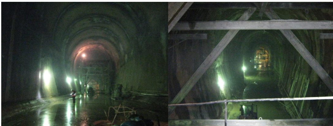
Figure 4-5 : DT1 tunnel, repaired sections in correspondence of the collapsed area–fault 35
