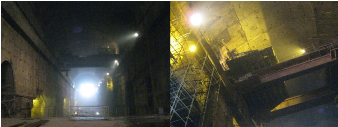
Figure 4-2 : Power house cavern on the left: View taken from the erection bay, on the right the installed overhead travelling crane
