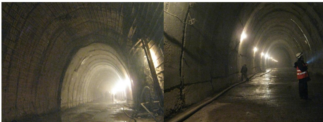
Figure 4-4 : Cable galleries, view from the transformer hall
