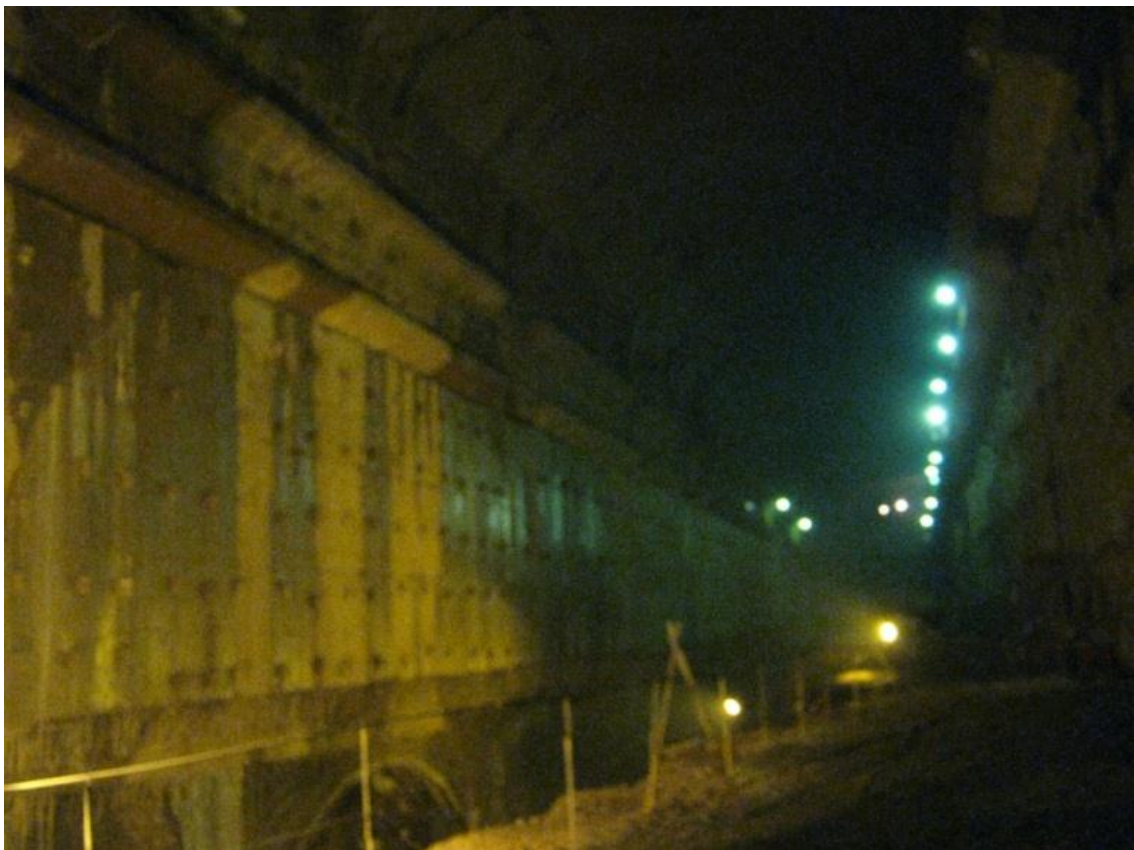
Figure 4-3 : Transformer hall cavern, upstream wall, view from Unit n 6
