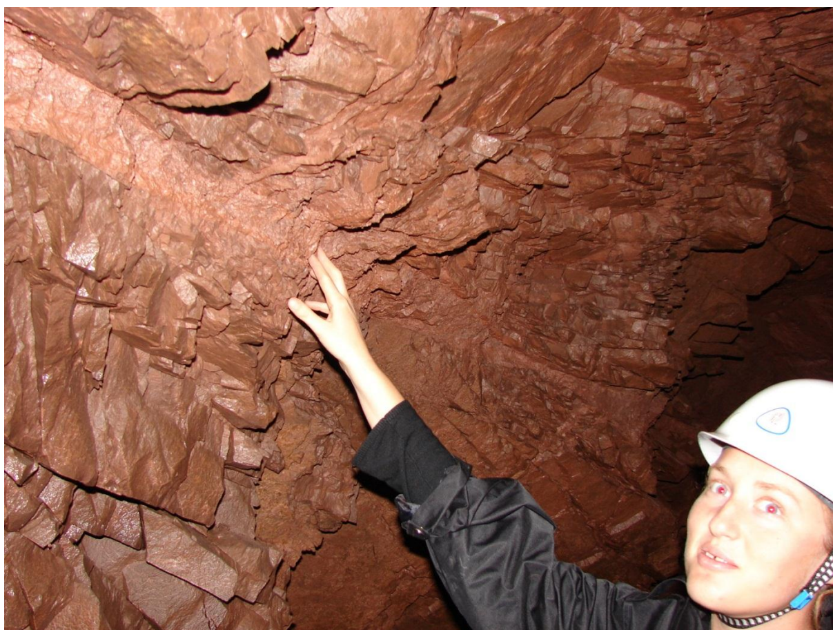
Figure 8.4: Kyzyltash Formation in investigation gallery 1030; one will note the subhorizontal joint with clay infilling and general dampness of the rock
