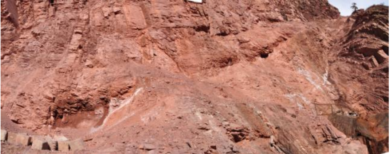
Illustration no. 22. Fault #35 in the Left Abutment of the dam.
