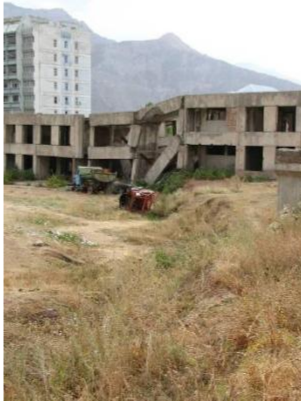
Illustration no. 45. Surface sinking causing damage to the buildings.
