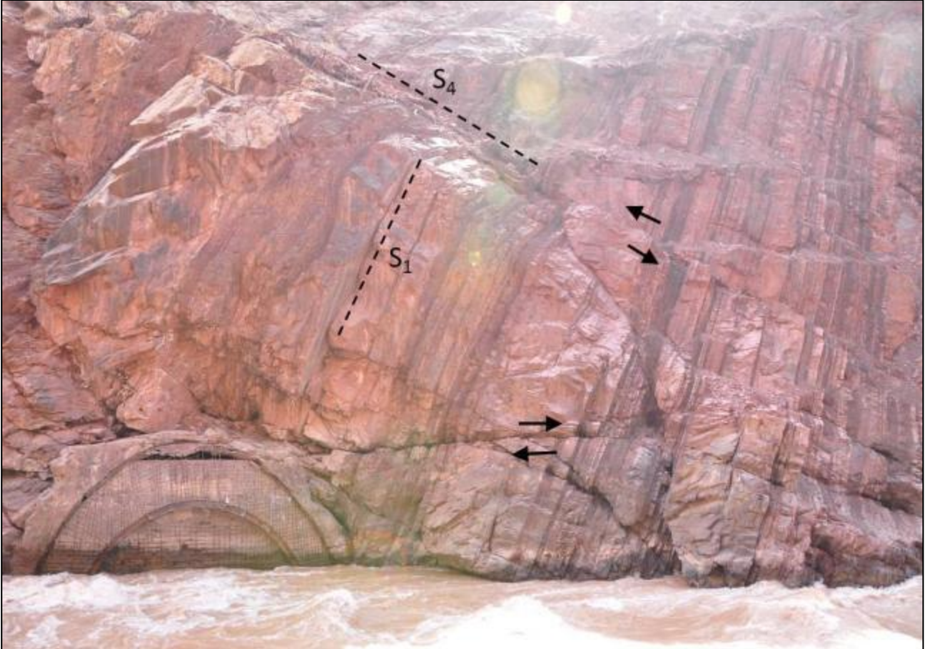
Illustration no. 26. Conspicuous joint sets at the dam site (here, in the lower part of the Right Bank).
