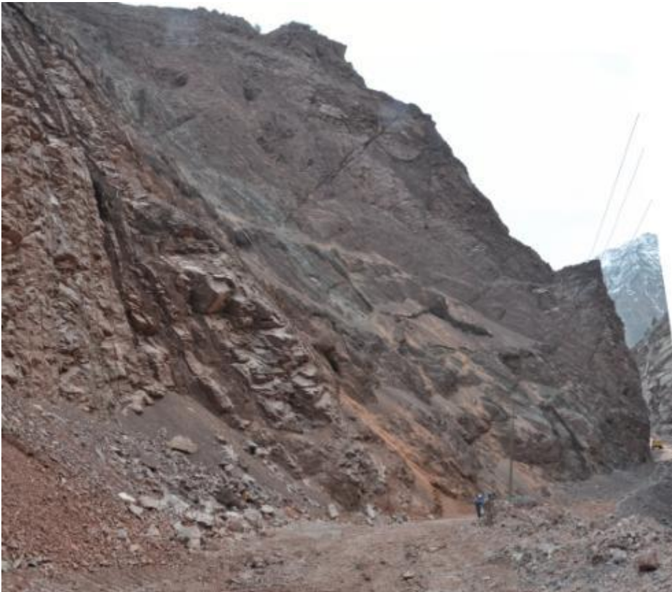
Illustration no. 24. Discontinuities of F#35 family, dipping upstream, in the Left Abutment.
