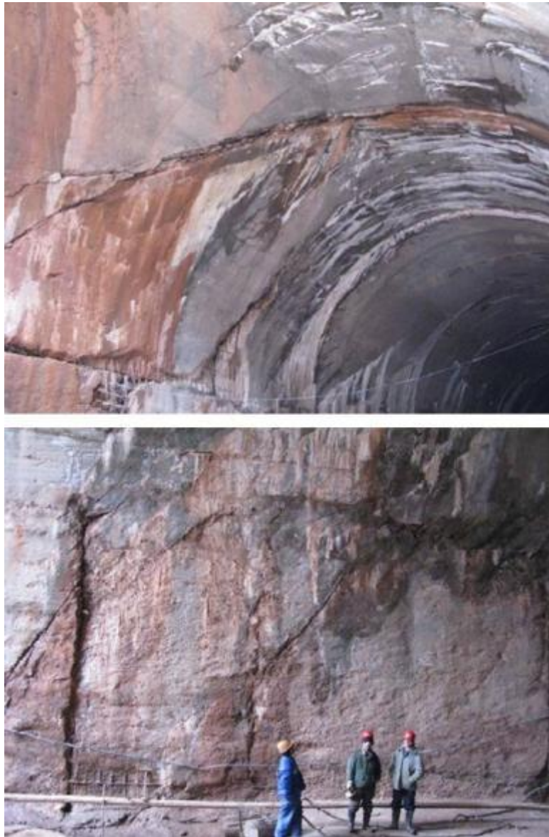
Illustration no. 44. Shearing of concrete lining and opening of construction joint in Diversion Tunnels I (above) and II (bottom).
