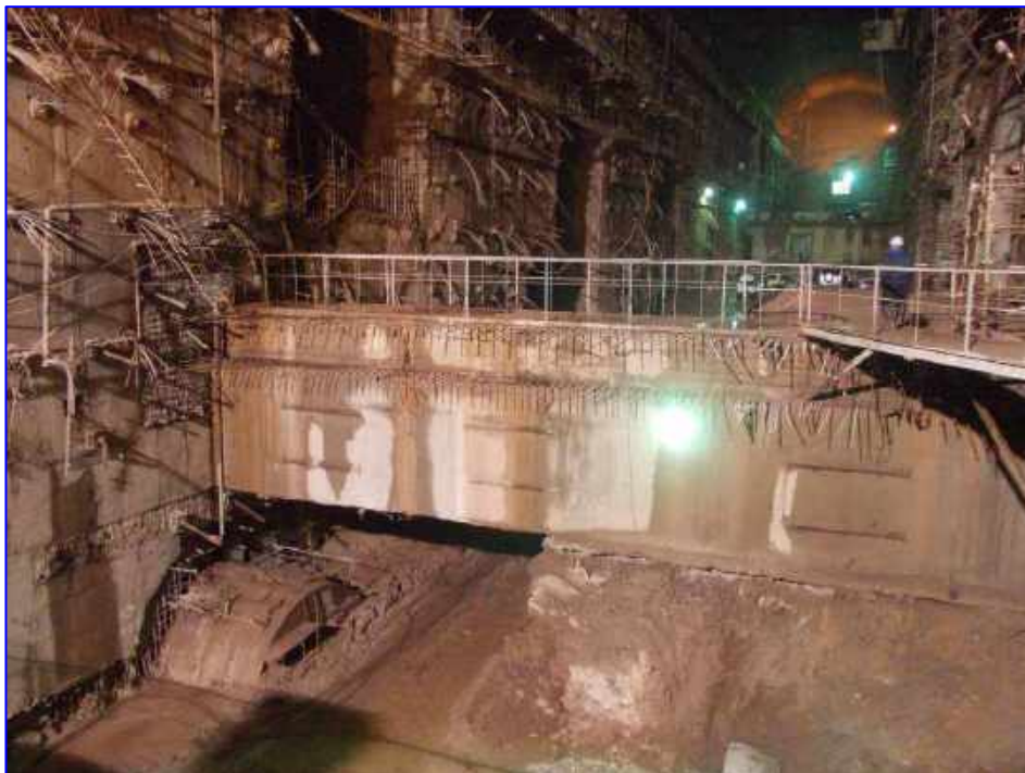
Figure 9: Photograph of reinforced concrete strut 2 between Units 6 and 5 (taken during the site visit of April 4-6 2013)
